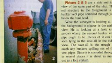
This is a Singapore flag container feeder vessel built in 1977. Picture 1 shows a surveyor peeling off a corroded eye.
